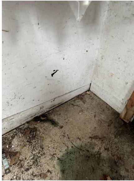
Figure 11 – Northeast corner from the interior – note how the walls have settled / rotted down around the slab
