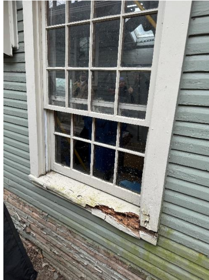
Figure 7 – Rotted window at north wall
