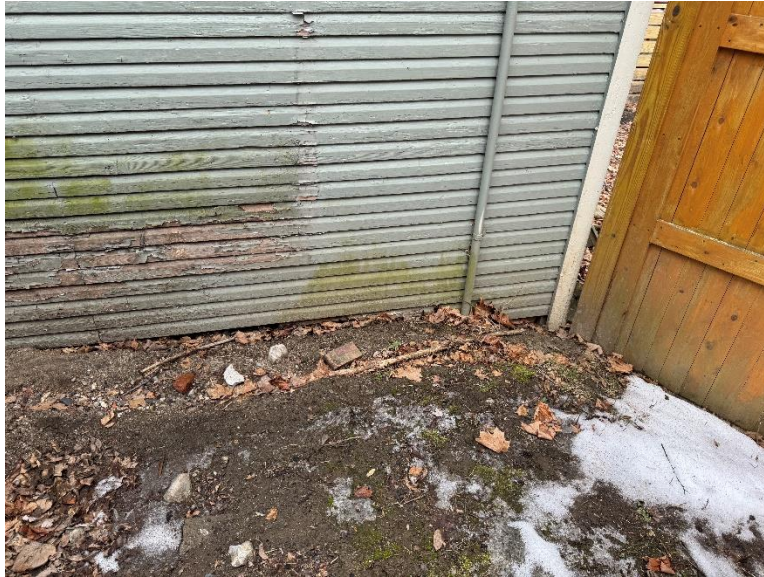
Figure 3 – Note base of wall sitting and below grade on north wall
