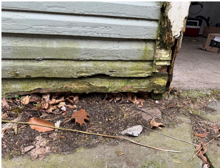
Figure 6 – Rotted framing and siding at entry door
