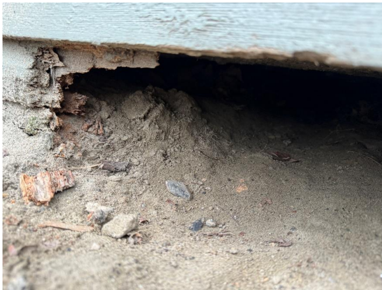
Figure 10 – Closeup of burrow undermined slab on west wall
