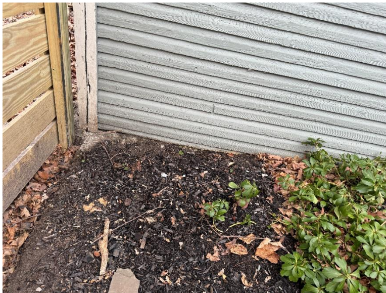
Figure 4 - Note base of wall sitting and below grade on south wall
