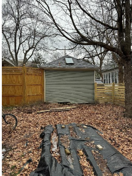
Figure 9 – West wall – note undermined slab
