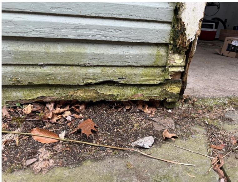
Figure 6 – Rotted framing and siding at entry door
