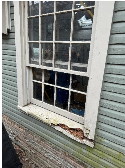
Figure 7 – Rotted window at north wall
