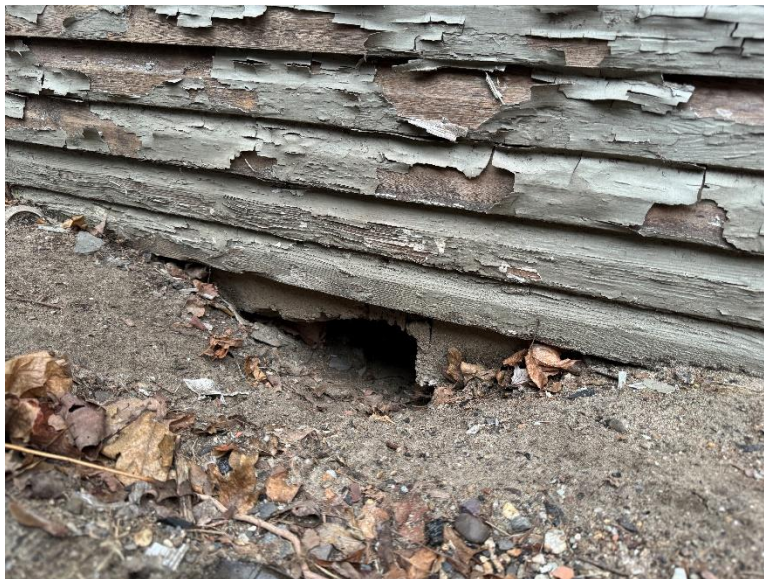
Figure 2 - Undermined slab and wood rot on north wall
